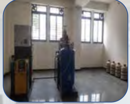
Liquid Nitrogen Plant
